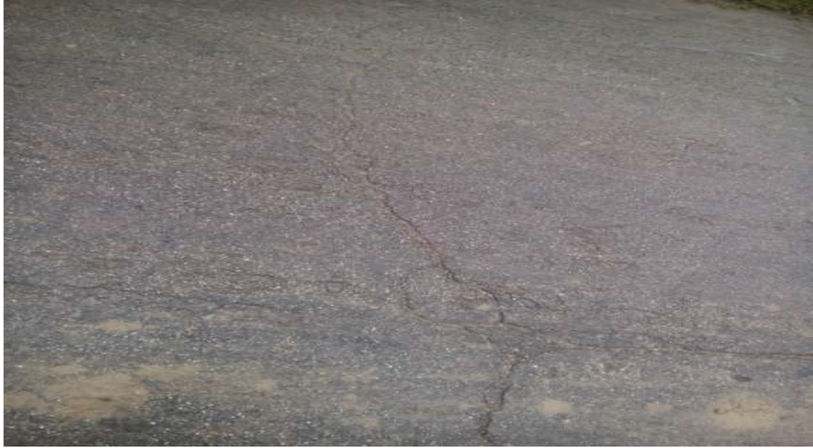
Plate 2.2: Photograph of Transverse Cracking (source:Field)
