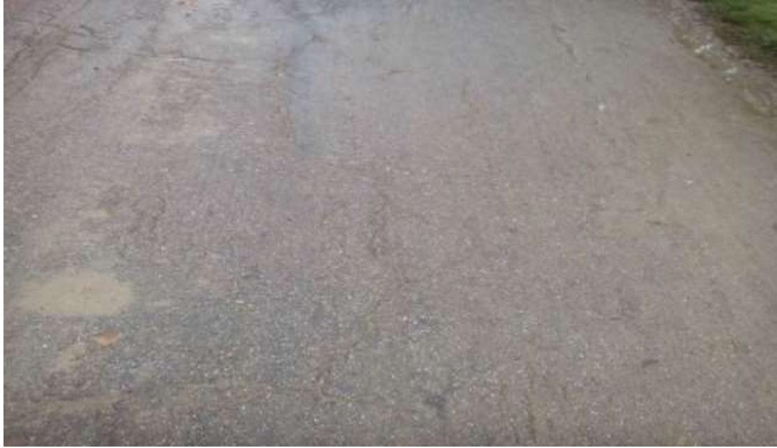
Plate 2.4: Photograph of Longitudinal Cracking (Mehedi and Mohd,2020).
