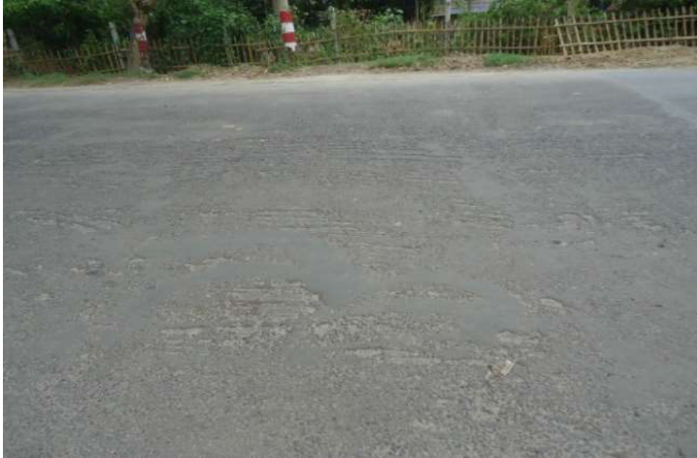
Plate 2.5: Photograph of Slippage Cracking (Mehedi and Mohd,2020).
