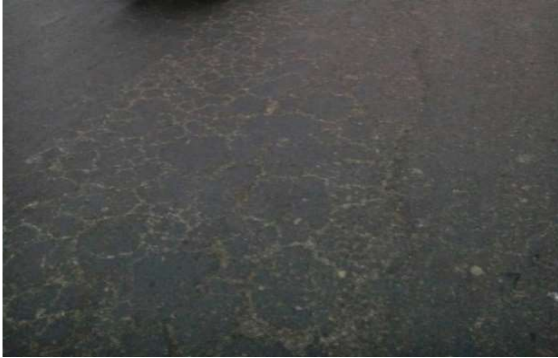
Plate 2.3: Photograph of Block Cracking (Mehedi and Mohd,2020).
