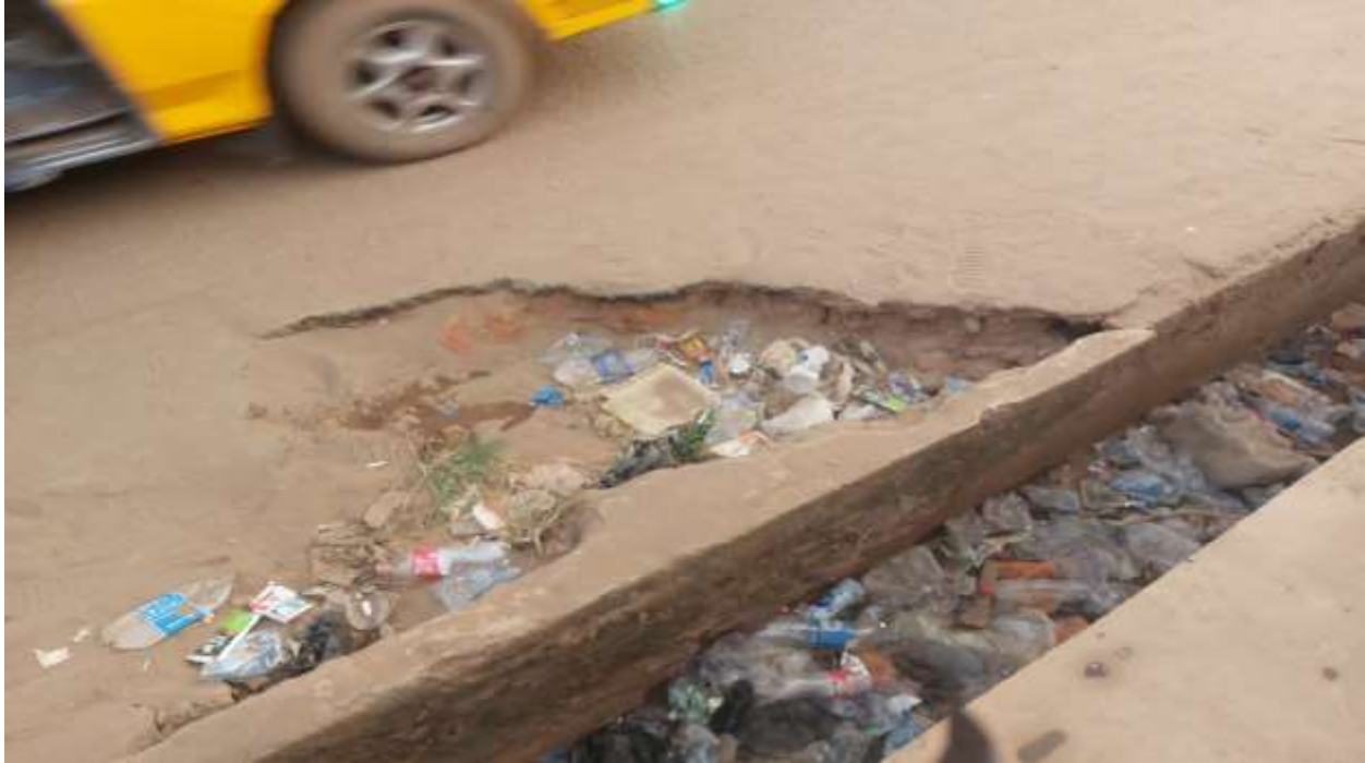
Plate 2.7: Photograph of Pothole along miracle junction ifite road (source: Field).
